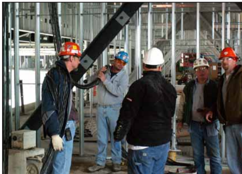
Telcom Services Installation (TSI) of St. Charles, Missouri is the installer of the ballpark's high-tech audio/video system, which reaches into virtually every corner of the stadium premises.
