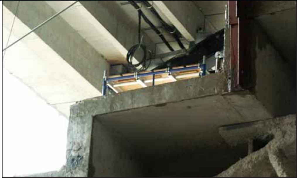
Belden YR46889 (P/N) Speaker Cables were used to provide optimal sound quality and integrity to the big speakers in the stadium's public address system. The cables are secured within the infrastructure by a J-hook two-hole strap.
